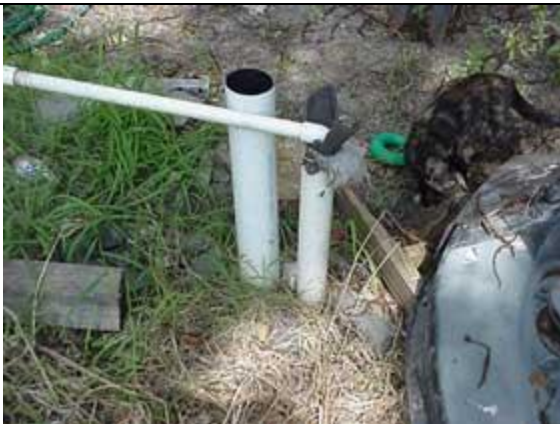
Picture 3. Abandoned well PVC casing. No annular cement or surface completion.
