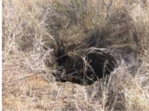
Picture 2. Abandoned well open hole
