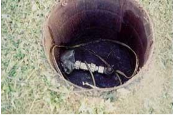
Picture 1. Abandoned well w/casing and pump
