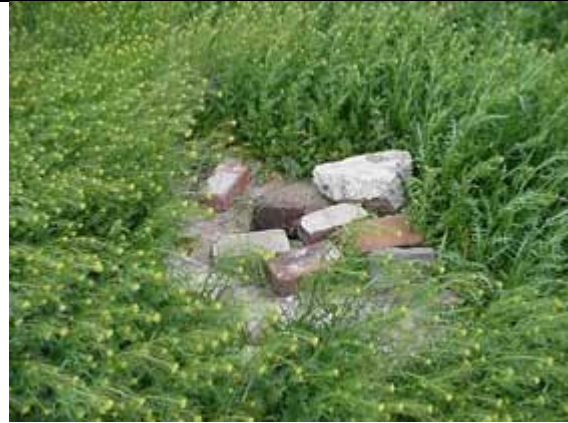
Picture 6. Capped abandoned well with deteriorated casing
